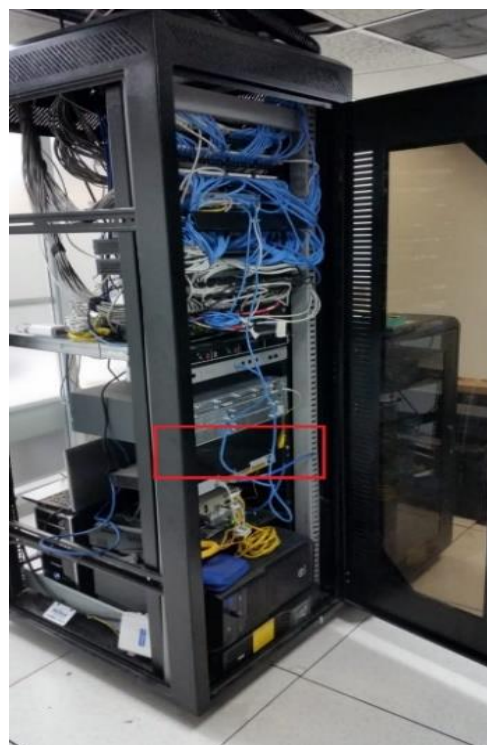
Figura 14: Rack servidores Novell Colombia.
