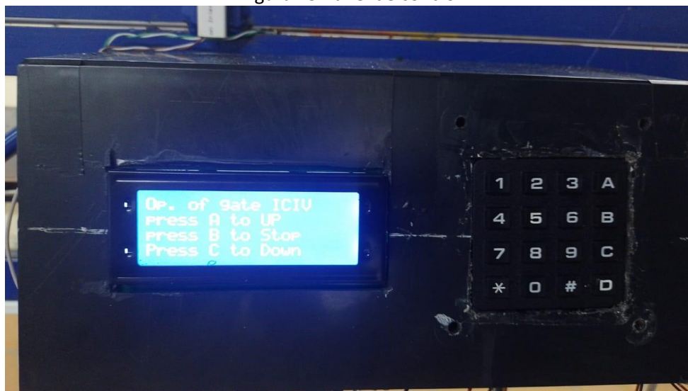
Figura 19 Panel de control
